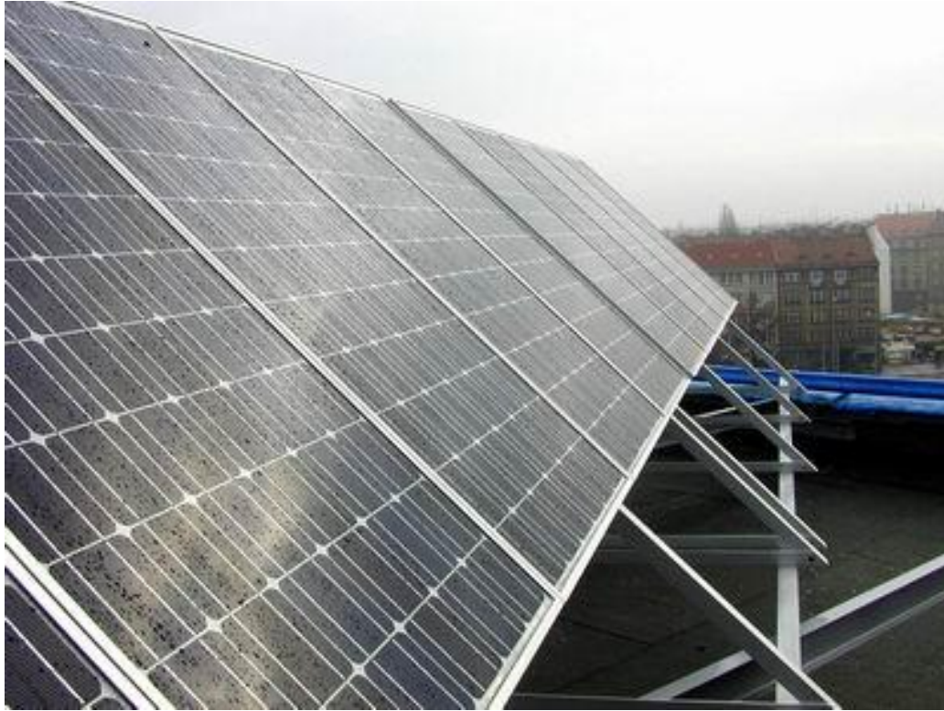
Fig. 3. The installed PV system on FEE CTU in Prague
