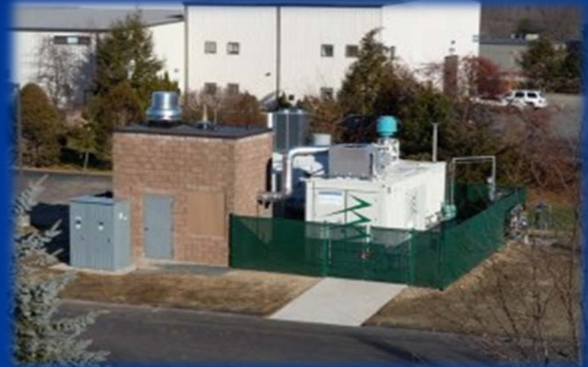
300 kW DFC300 fuel cell power plant, Fuel Cell Energy
